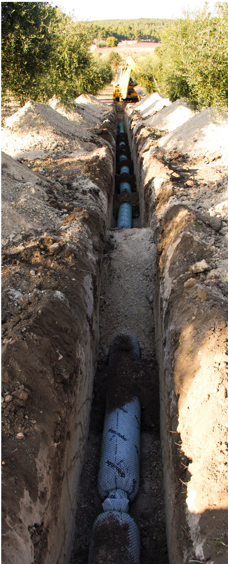
Drainage agricole — Fontanars, Valencia
