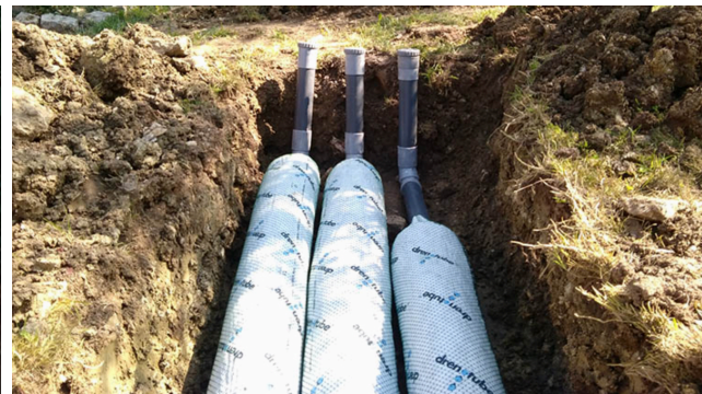
Wastewater treatment plant installed in Opio, France
